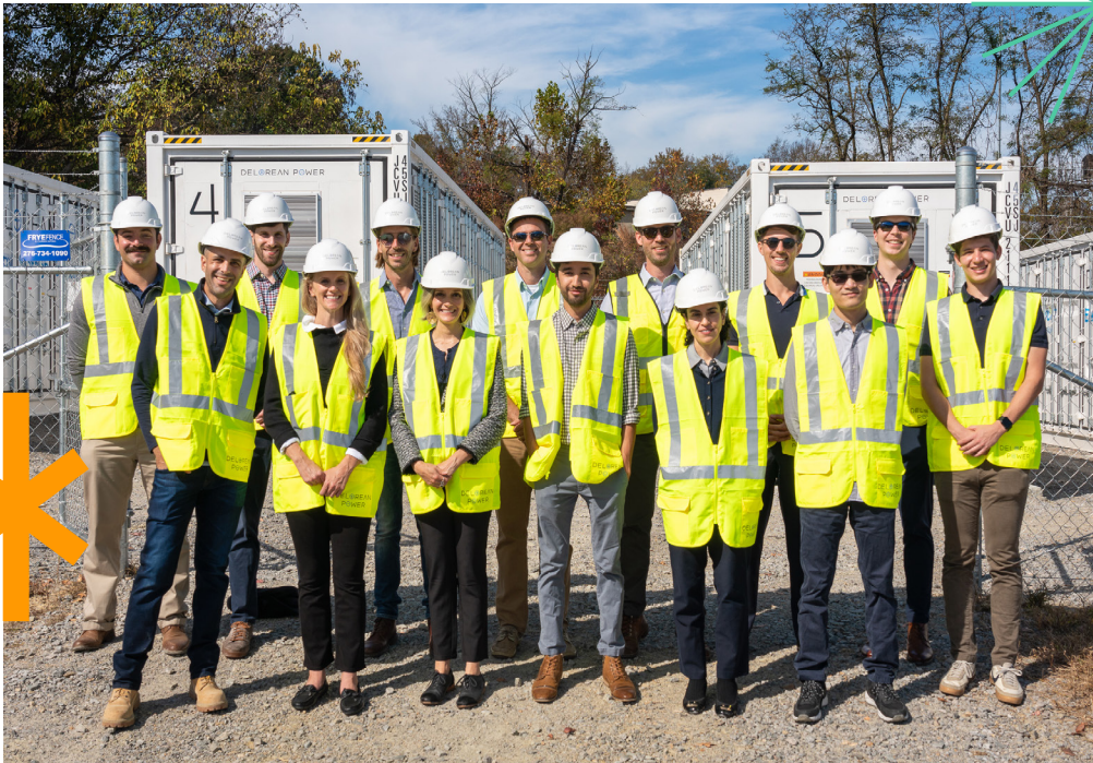
Delorean Power team at the groundbreaking of their 25 MWh battery storage installation in Danville, VA
